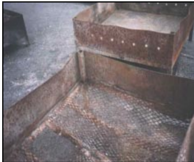
Note the warping of the steel from burning operations. Also note debris on ground surrounding pan - evidence of kickout or spillage of ash.
